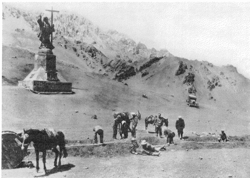
Symbol of Neighborliness in South America. At the feet of Christ of the Andes, I. T. & T. engineers and installers burying the transcontinental cable interconnecting Argentina and Chile.
