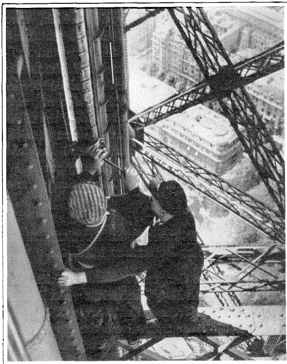
Special Coaxial Cable Connecting the Eiffel Tower Television Transmitter with the Aerial at the Top of the Tower. The cable met rigid frequency characteristic and low attenuation loss requirements; it spanned the distance of over 380 metres between the transmitter and the aerial and weighed 12 tons.
