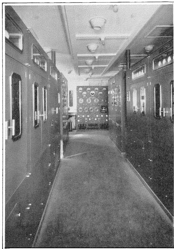
"Queen Mary" Radio Transmitter Room, Showing the Transmitters Remotely Controlled from the Radio Operating Room 400 Feet Away.
